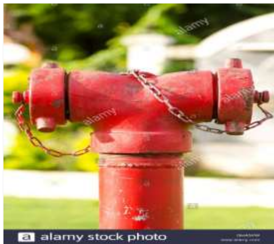
FIRE HYDRANT HOSE CONNECTION FIRE FIGHTING
